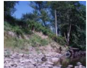
North Edge of Pilchuck Creek Embankment Failure
