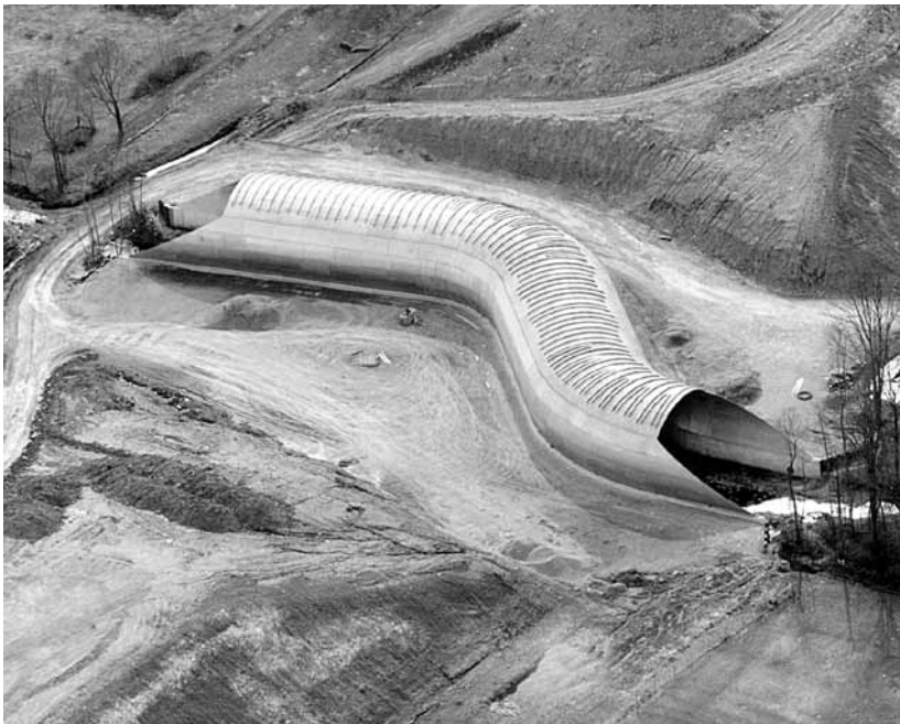
High-profile arch SUPER-SPAN (43'-3" span, 27' rise) in Hamilton, Ohio to span a wetland and to provide a wildlife crossing.
