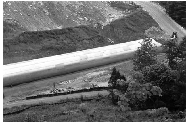
24'-0" diameter steel MULTI-PLATE® under 60 feet of fill owned by VDOT in Dryden, Virginia
